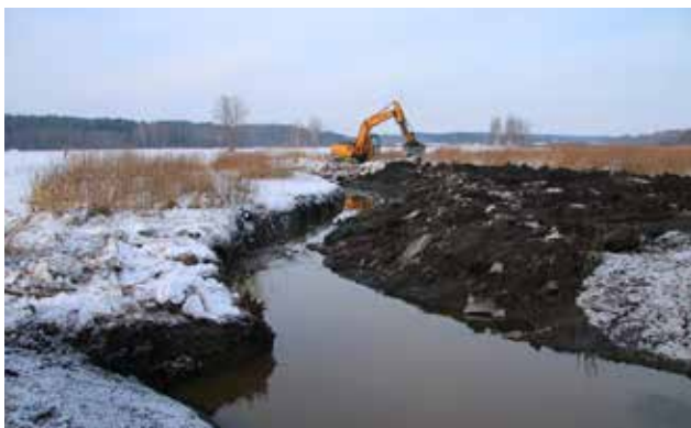
Figure 16. Excavation was performed mainly from both banks of the old riverbed (30.01.2015; picture shows a half of the river's width excavated). Photo: I. Priedniece
