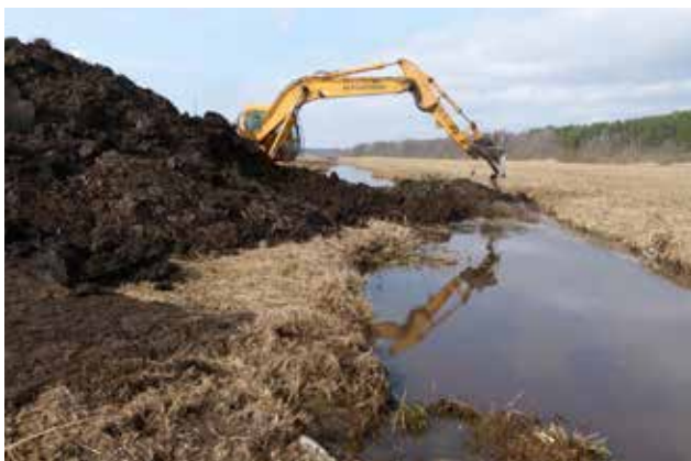
Figure 23. Construction of the second dam on the straightened riverbed (25.03.2015). Photo: E. Račinskis
