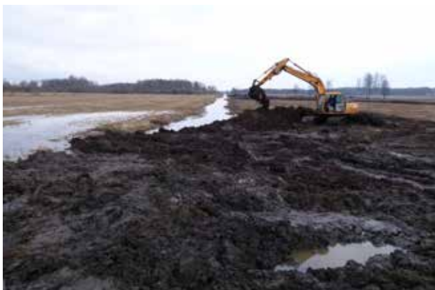
Figure 21. Construction of the first dam at the upper part of the restored section (05.03.2015). Photo: E. Račinskis
