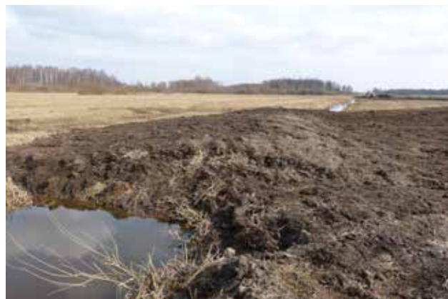
Figure 22. The first dam at the upper part of the restored section completed (25.03.2015). Photo: E. Račinskis
