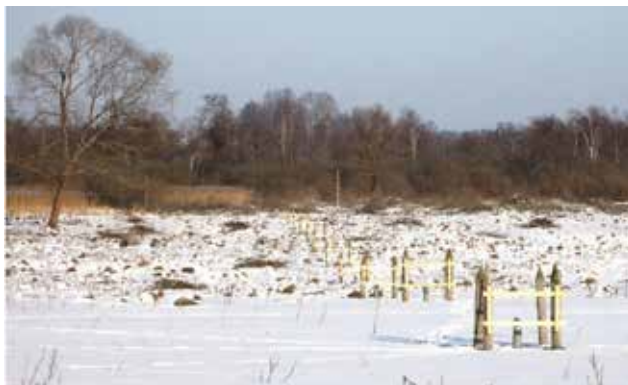
Figure 3. The new groundwater monitoring wells in January 2012 (Photo: D. Gruberts)
