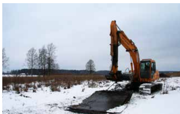
Figure 18. In most sloughy sites metal plates were put under the caterpillars of the excavator (29.01.2015). Photo: I. Priedniece
