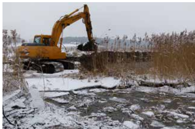
Figure 15. River restoration was carried out in winter in order to harm nature as little as possible and to ease working with the excavator in the sloughy floodplain (23.01.2015). Photo: E. Račinskis
